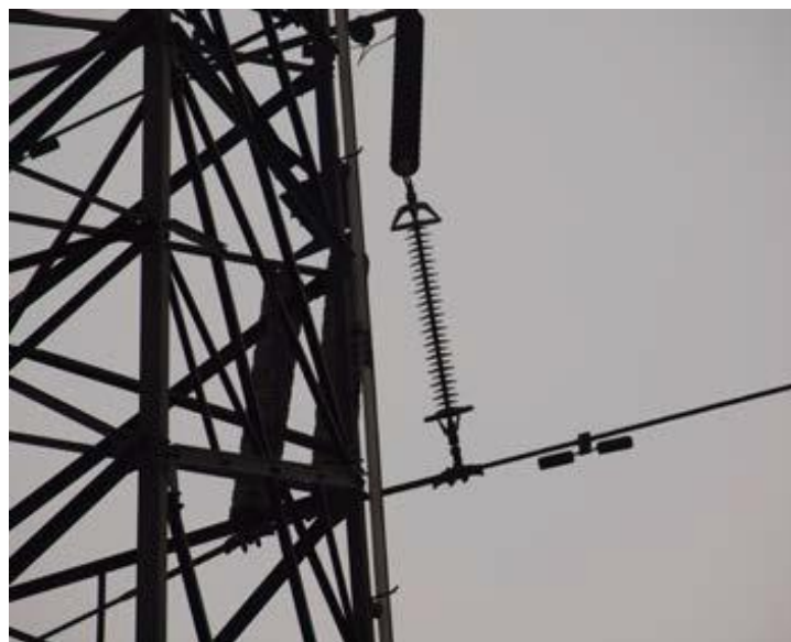
Figure 7: the transmission line lightning arrester
